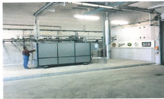
Figure 33 - CHP Plant/Power station. Supplier of the technology: Thermic Energy RZ GmbH
